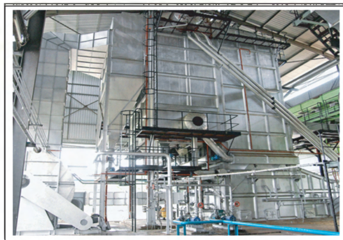
Picture of an installed and commissioned boiler
